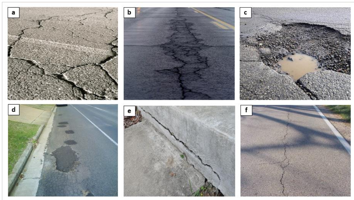
Figure 4. Examples of distressed pavement in Malaysia (a) shattered cracks; (b) surface deteriorations; (c) potholes; (d) road patching; (e) corner cracks; (f) longitudinal cracking.
